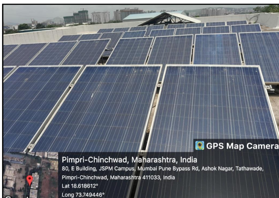
Photograph of Roof Top Solar PV Plant:
